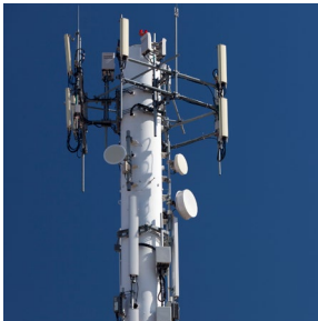
Cellular Base Stations
